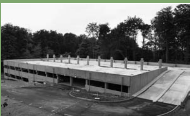
Step 5: Build a ramp. Et voilà, you have brand new carpark with two decks, 250 places and a maximum headroom of 2.1m (watch out, Rob and Carsten)...
